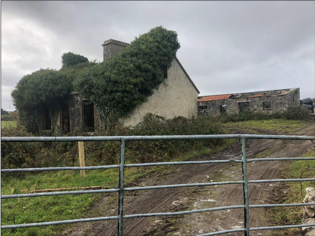
Plate 1: Existing derelict dwelling and outbuildings (to be demolished) located in the south east corner of the application site (Photo: MKO)
