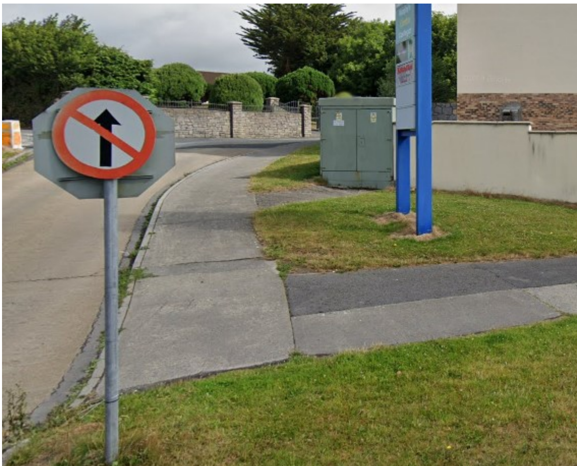
Fig 1: Existing Ground Mounted Sub Station for medium voltage connection
