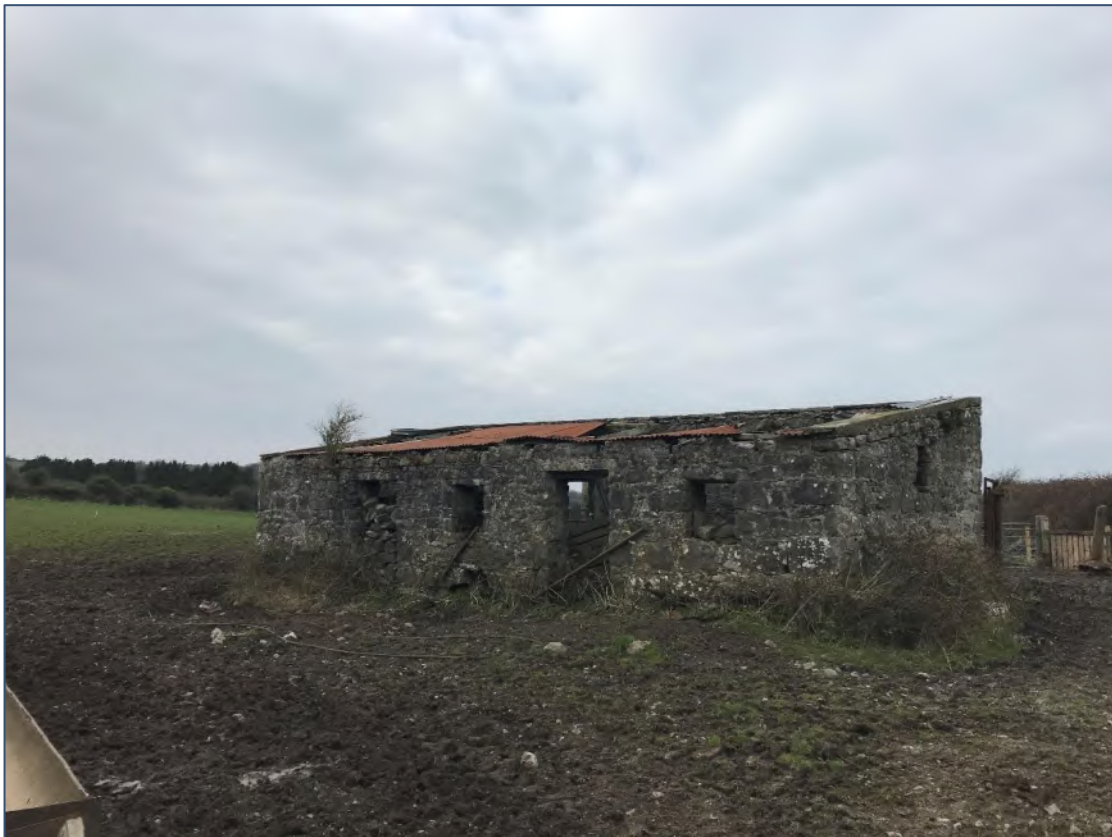
Plate 2-3 Sheds occur to the north of the cottage, used for agricultural purposes, and surrounded by Spoil and bare ground (ED2), associated with livestock poaching.
