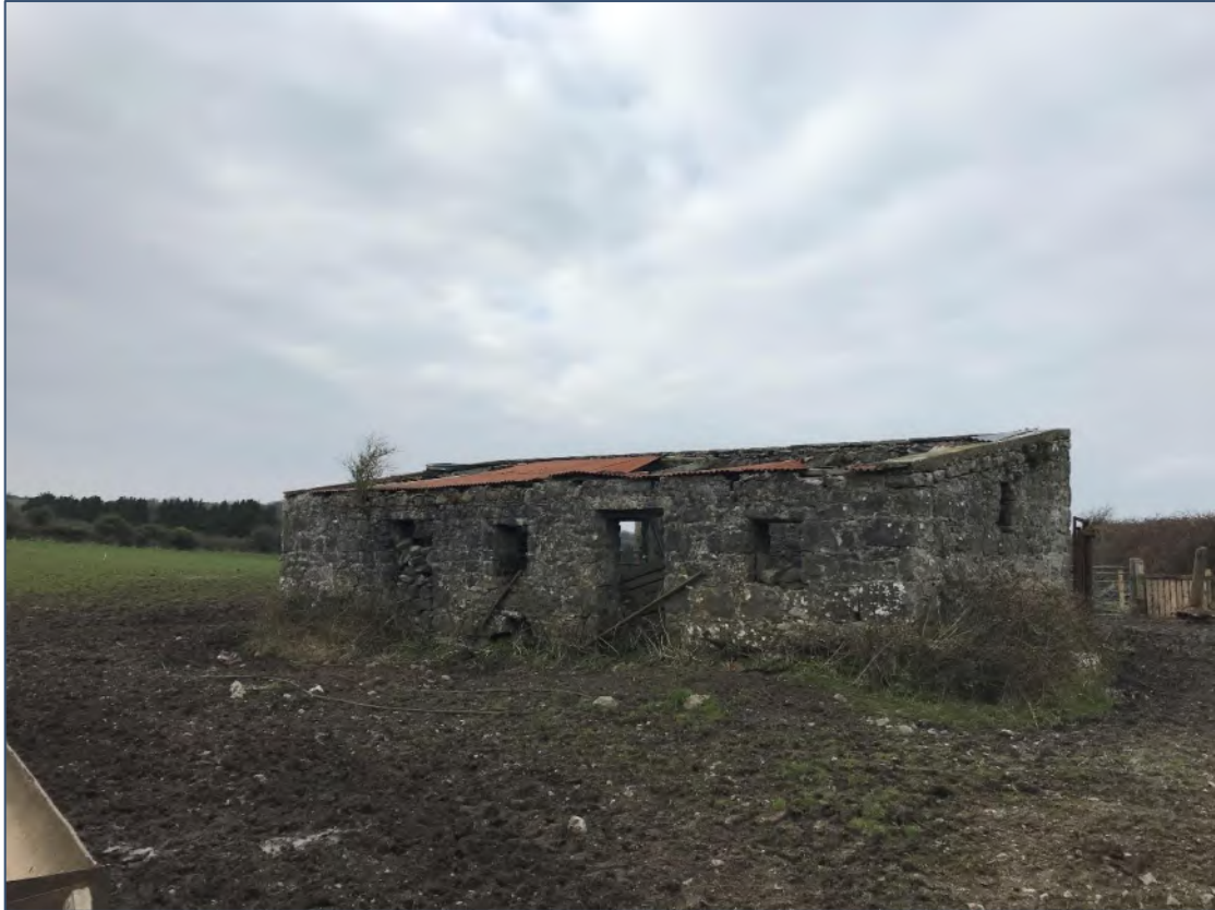
Plate 5-3 Sheds occur to the north of the cottage, used for agricultural purposes, and surrounded by Spoil and bare ground (ED2), associated with livestock poaching.
